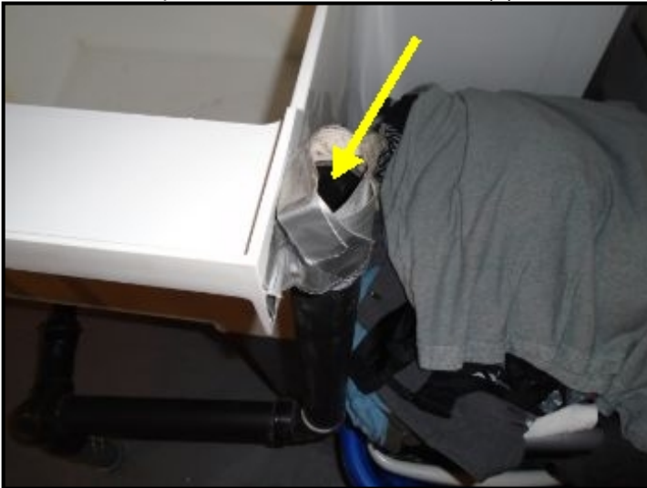
An air admittance valve should be added to the sewer drain line at the basement sink (2).
