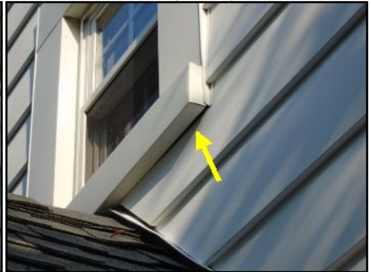
Repair all gaps in siding to prevent moisture / pest entry (2).
