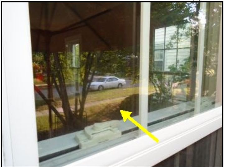
Fog/condensation observed at the front left and front right windows which is an indication of a failed seal (2).
