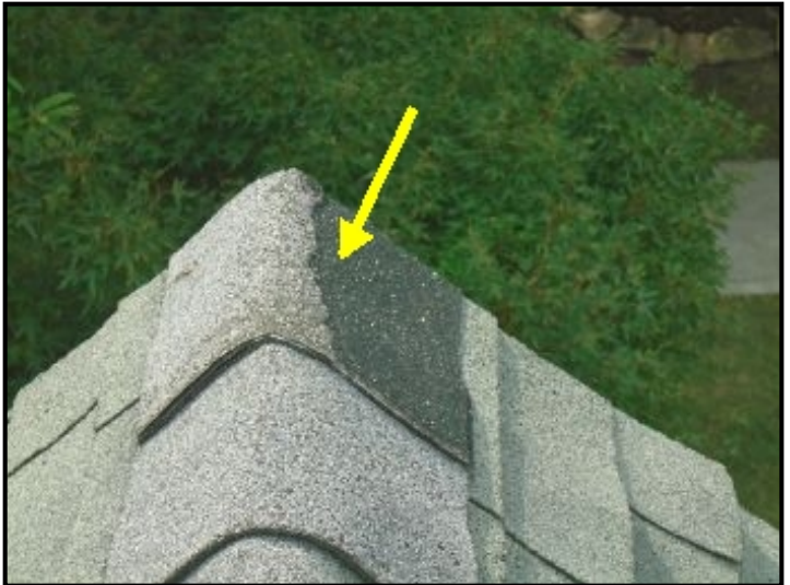
Overall, roof is in marginal condition with several shingles showing signs of significant deterioration and surface wear (1). Significant curling and cupping of the shingles were observed in several locations (1).
