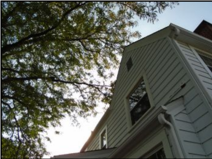
Trim back tree branches that overhang the roof to prevent damage / wear on the roof (2).
