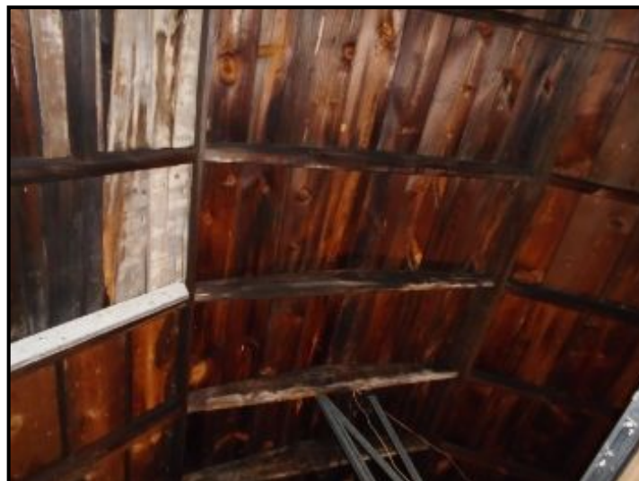
Water stains / water damage observed on roof framing indicating previous roof leaks (1). Repair any damaged boards that are rotted or weakened (2).
