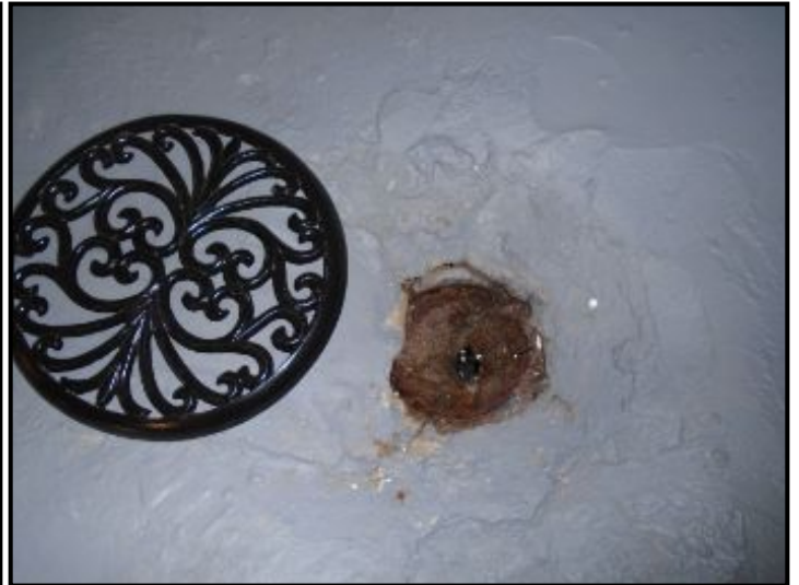
Basement floor drain has corroded significantly (2).
