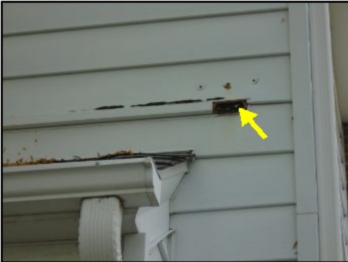
Remove exposed wiring and junction box at rear of house and repair siding as needed (2).
