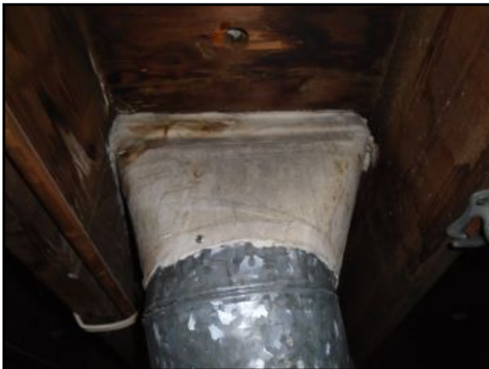
Possible asbestos materials observed at the HVAC ductwork (2). Laboratory testing must be performed to determine if asbestos is present in the ductwork insulation (2).
