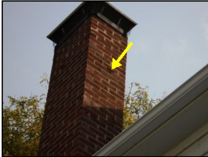
Some mortar deterioration observed at brick chimney requires tuck-pointing (2).
