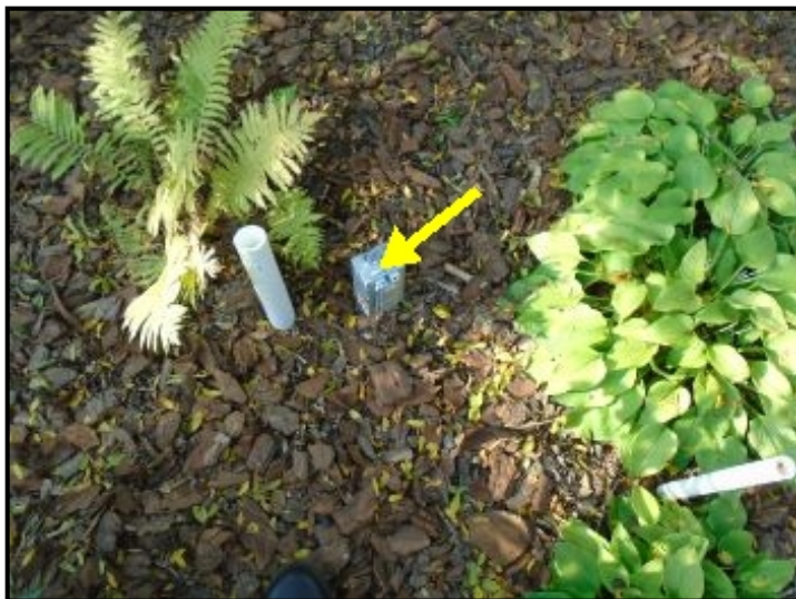
Exterior yard GFCI outlet test/reset buttons were not functioning (2).
