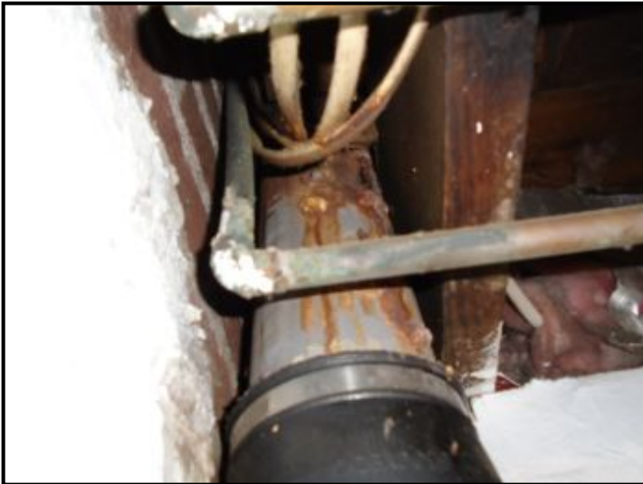
Corrosion / stains observed from previous leaks at the main drain line observed in basement (1). No current leaks observed; however, monitor for leaks and repairs may be required to corroded metal drain (2).
