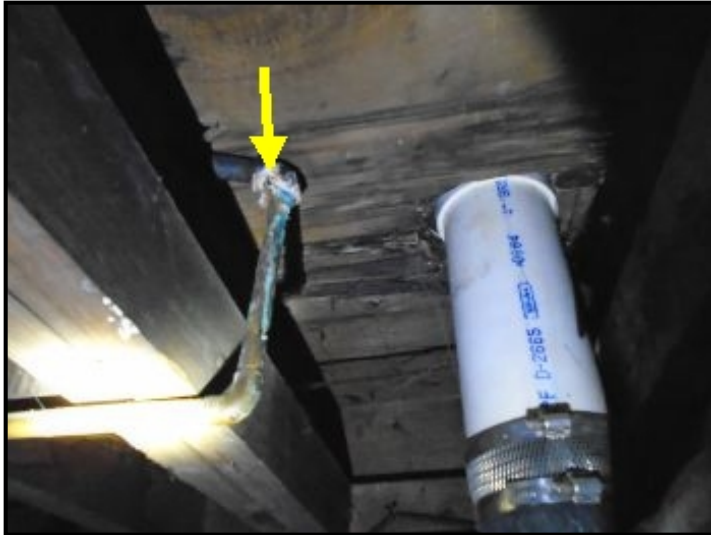
Corrosion observed on copper water line in basement should be cleaned and monitored to ensure corrosion is not continuing (1).
