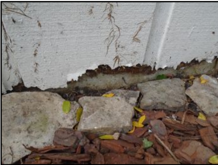
Garage wood siding and trim was in contact with the soil and rotted / termite damaged in several locations (2).
