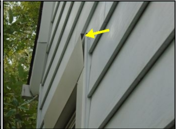
Loose siding needs refastened at front right side (2).
