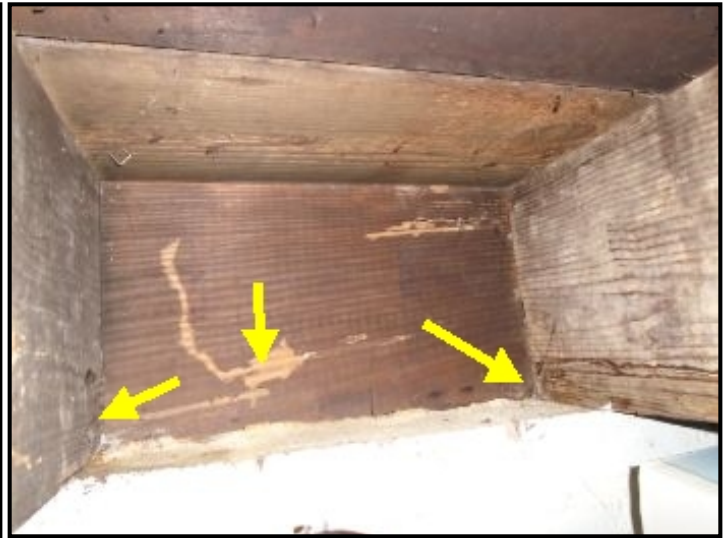
Termite damage to the wood floor joists and framing on top of the front foundation wall was observed in the basement; however, no current signs of active infestation was observed (1).
