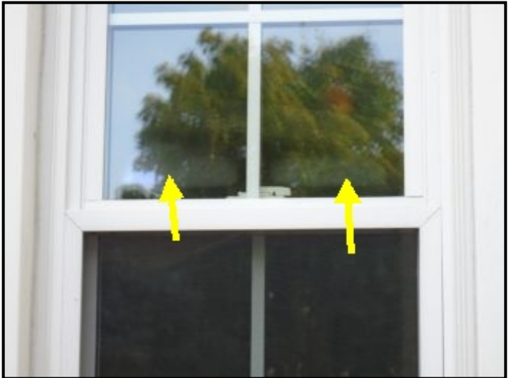
Fog/condensation observed at the front left and front right windows which is an indication of a failed seal (2).
