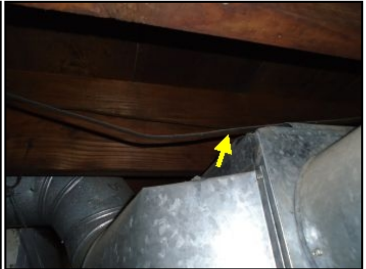
Knob and tube conductor was sagging and resting on the HVAC duct work which could energize the duct system if any insulation is damaged and exposing the copper conductor (2).
