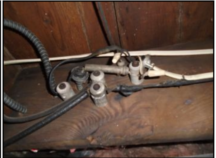
This property has "knob and tube" wiring which was commonly installed prior to 1950. It is ungrounded and considered unsafe by today's standards (2). Over time, the wire's insulation becomes brittle and falls apart, resulting in exposed conductors and a risk of shock and/or fire (2). A qualified electrician should replace the wiring as necessary (2). Knob and tube wiring was observed in the basement, attic, and through the walls as seen at several outlets at the first floor and upstairs bedrooms (2). Recommend replacement of any other ungrounded cables including metallic sheathed cables as required (2). Recommend GFCI outlets in Kitchens, Bathrooms, Garage, Laundry Area, Exterior, and other required areas (2). Upgrade outdated lights switches and outlets (2).
