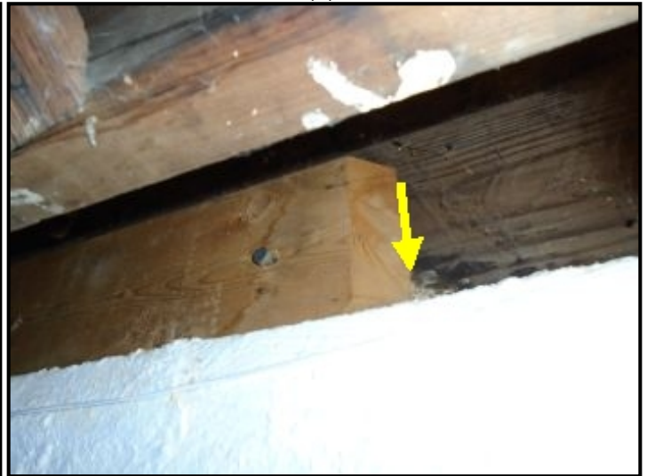
Repair to joist on top of foundation wall observed near gas meter may have been due to previous termite damage; however, damaged wood was covered by the new wood splice (1). No current signs of active infestation were observed (1).
