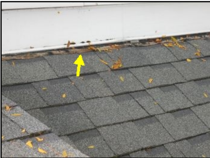
Flashing beginning to rust / deteriorate in several locations (2).
