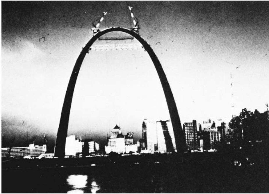
FIGURE 1. Construction of St. Louis Gateway Arch. (Copyright© American Institute of Steel Construction, Inc. Reprinted with permission. All rights reserved.)
